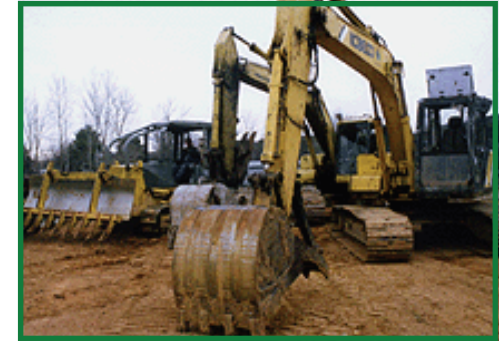
Typical grading violations include clearing vegetation on slopes, having large equipment on site that is altering the landform and/or impacting existing drainage conditions, and/or depositing or excavating soil on site.
